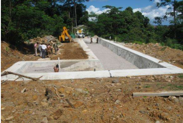
An L-Shape constructed wetland at Mahe, Seychelles. The design was adopted to meet the space requirement.
