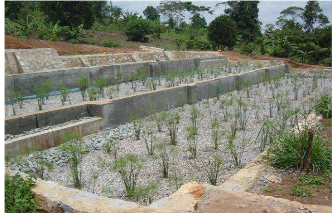
Sloping constructed wetland system at Seeta School, Uganda, the design was adopted to meet the requirement of sloping terrain.
