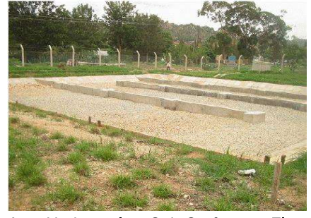
A Horizontal Sub-Surface Flow Constructed Wetland with baffles to improve the retention time and thus treatment performance.
