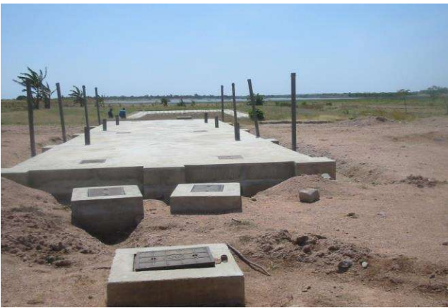
A combination of Septic Tank and Constructed Wetland at Bariadi Prison in Tanzania
