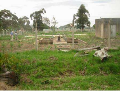
Malfunctioning mechanical aeration, wastewater treatment system at Kleruu Teachers' Training College in Tanzania.
